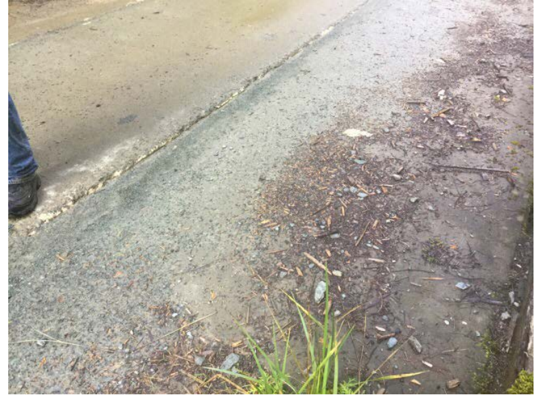
Upstream slab settled by approx 1" on upstream. Monitor.
